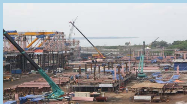
Process Gas Compressor Module
