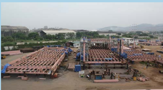
Turbine Generator Module
